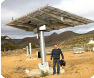
Searl Derman with one of the installations.
