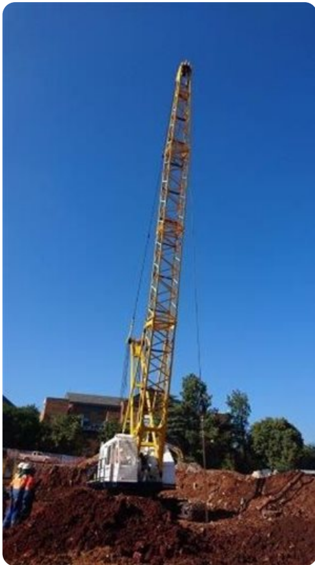
Aecom encountered challenging dolomitic ground conditions at the Exxaro head office site in Centurion.
