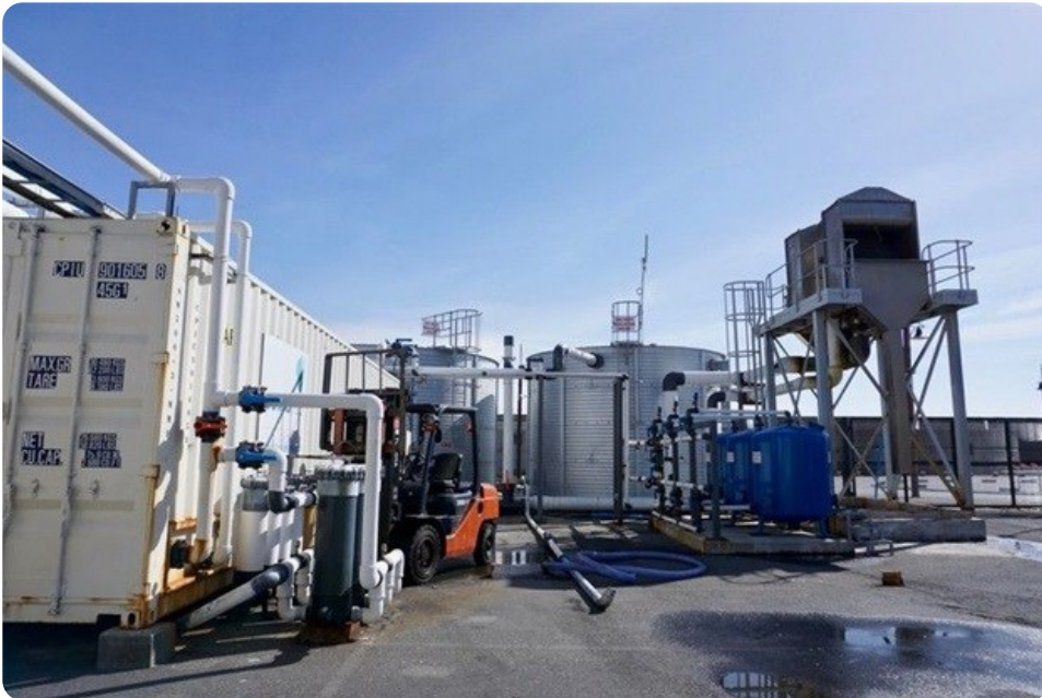
Quality Filtration Systems runs this desalination plant in the Waterfront. Photo: Kristine Liao
