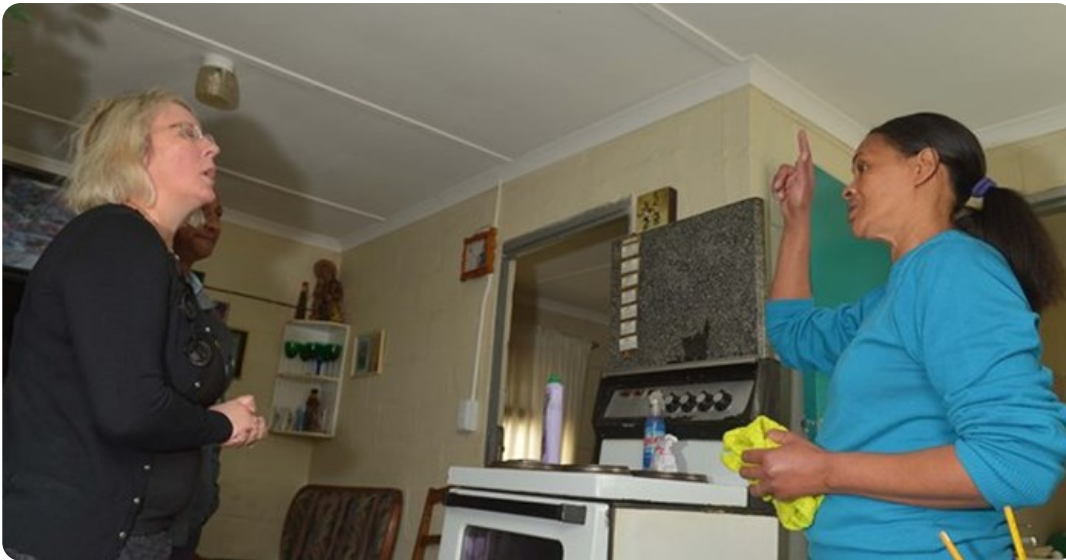
Councillor Van Minnen inspects the ceiling of Mrs Jennifer Jonas in Vrygrond.
